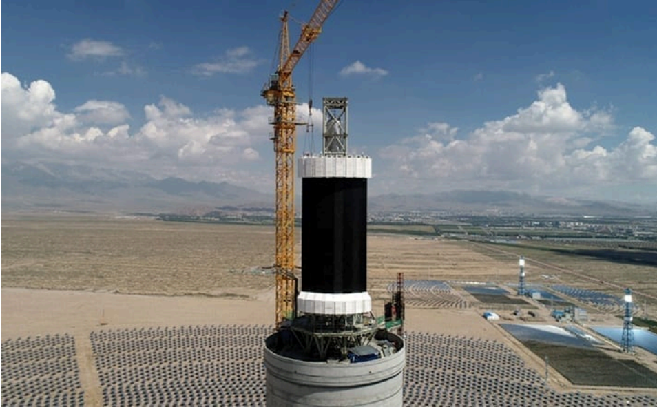
1. This image shows installation of the tower’s receiver, which is coated with specially formulated high-temperature black coating to increase absorptivity. Courtesy: Supcon Solar
